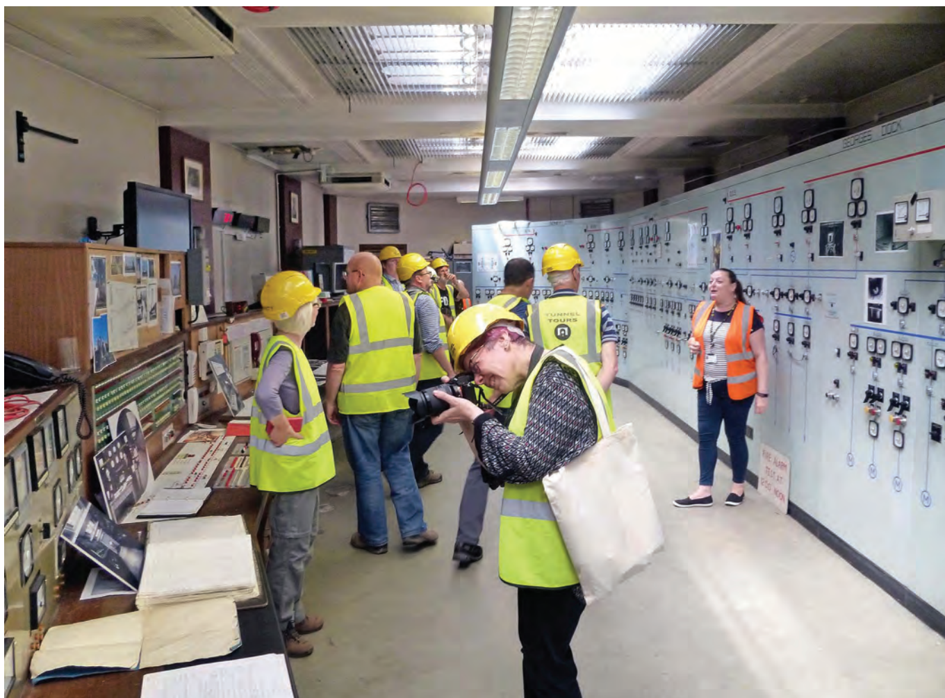
SubBritters looking at the 1930s control equipment for the Mersey Tunnel, high in the George's Dock building.
